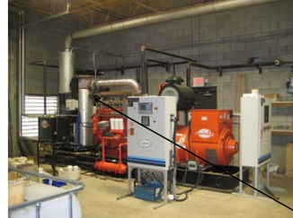
Modified diesel generator with thermal recovery for process heat →
