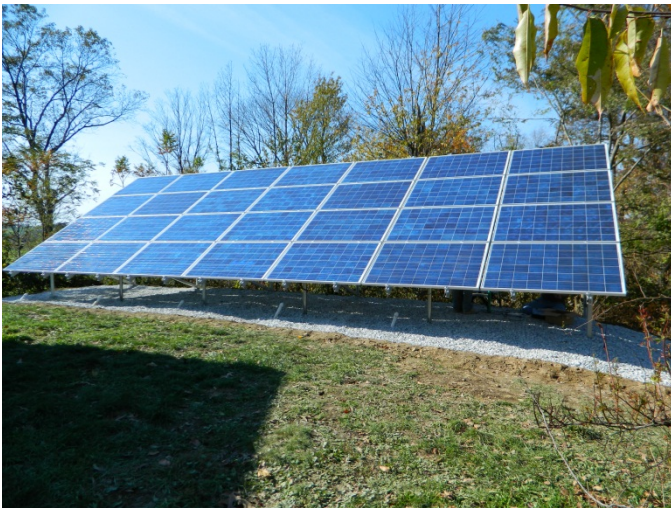
A ground mounted solar PV array
