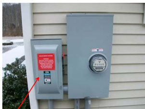
An outdoor, visible disconnect is required for solar PV systems
